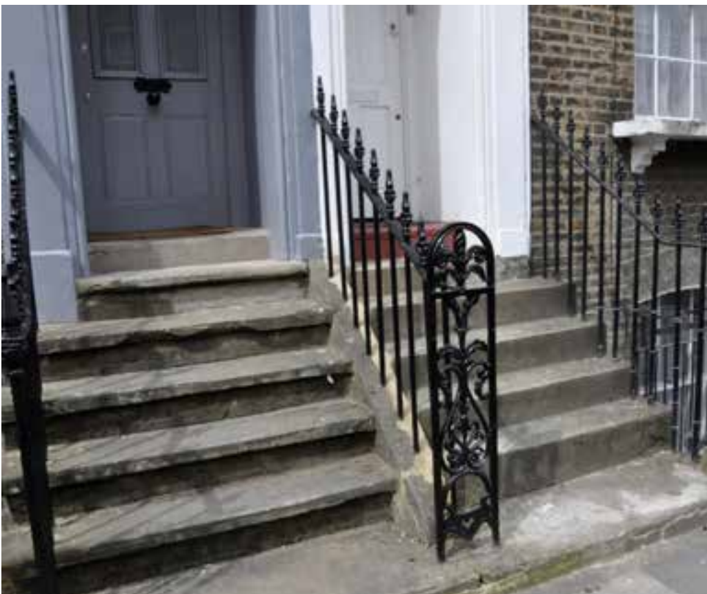
Below: Original wrought ironwork boot-scraper situated between two houses on Driffield Road. This design feature is also found on Grove Road. Also note, the loss of stone nosings to the modern steps on the right.
